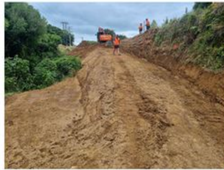
Figure 4: Opunake Road under slip – access ramp
