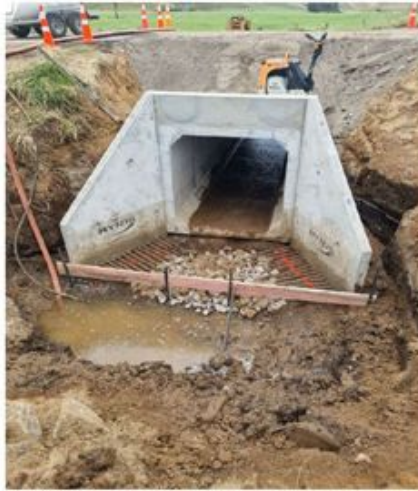
Figure 3: The new culvert installed under Wawiri Rd with temporary backfill over the culvert.
