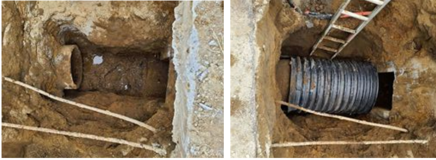
Figures 11 & 12: Collapsed Stormwater Tunnel Remediation Works
