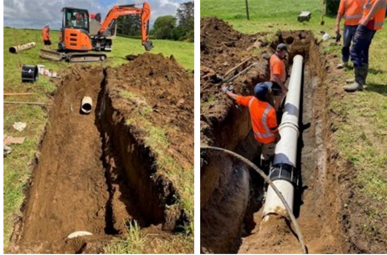
Figures 9 & 10: Trunk-main Break and Repair respectively
