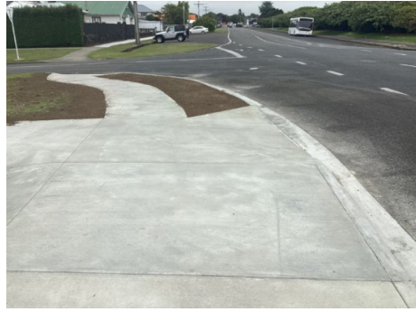
Figure 4: New Footpath on the south side of Fenton Street from Cordelia Street to Ariel Street.
