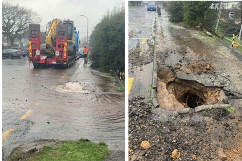
Figure 5: Romeo Street AC pipe break
