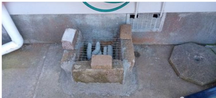
Figure 9: Illegal downpipe sewer connection and remedial works
