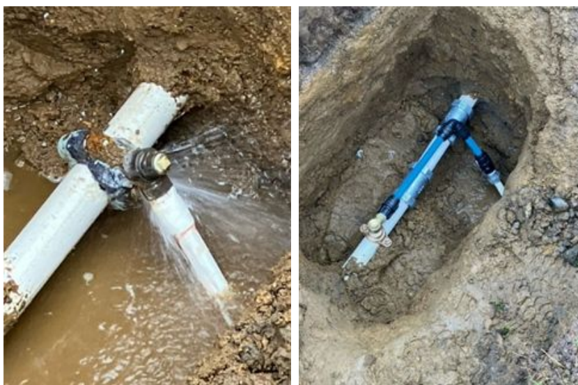
Figure 6: Leaking 50 mm PVC rider main tapping band and repair
