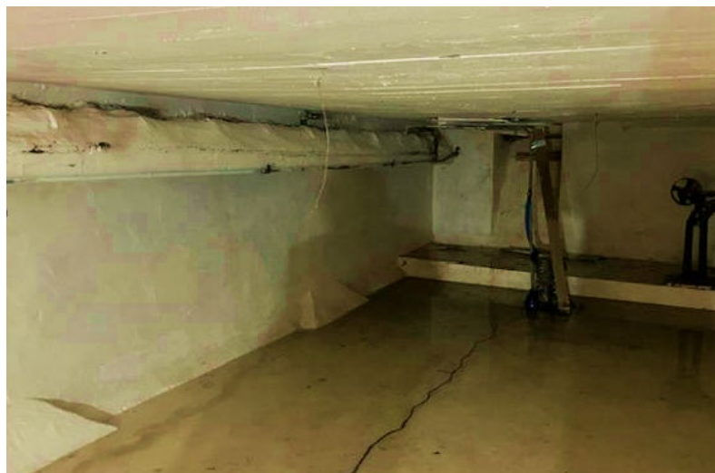
Figure 10: Storm water pipe location under Kings Theatre
