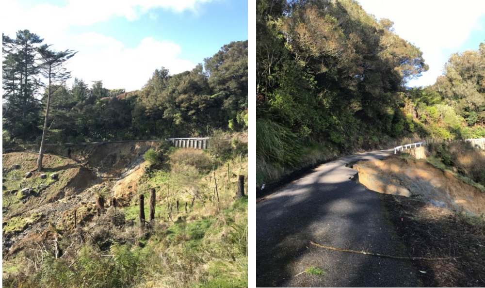
Mohakau Road Slip
