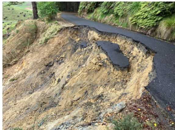
Figure 2: Figure 1: Major slip on Mohakau Road
