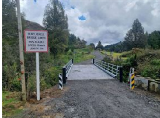
Figure 4: Completed concrete deck to replace the old wooden deck. Note the steel bollards on the approaches to the bridge.
