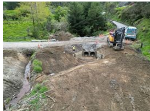
Figure 2: The new twin 900mm culverts replacing the two existing culverts. The concrete culvert to the left has been removed
