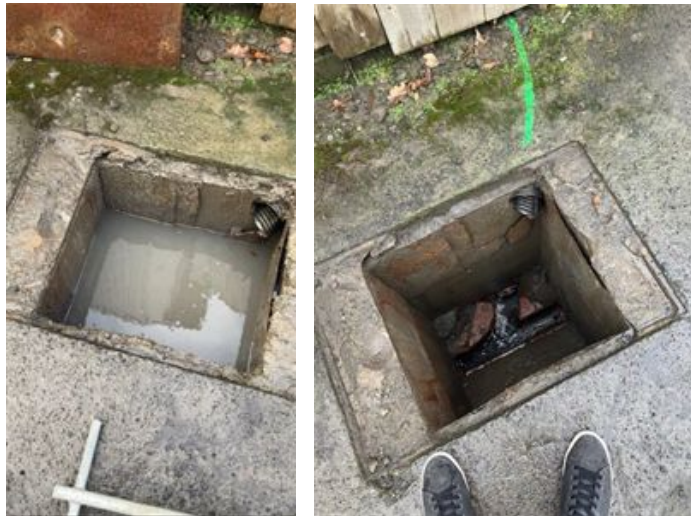
Figure 4: Drain connected to sewer overwhelmed during extreme rain event.
