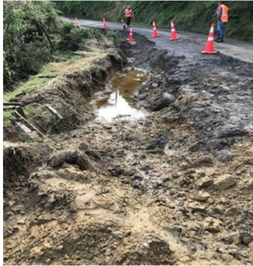
Figure 1: Damage to the roadside shoulder on Junction Rd. This has been repaired, with the costs being recovered from the forestry company.
