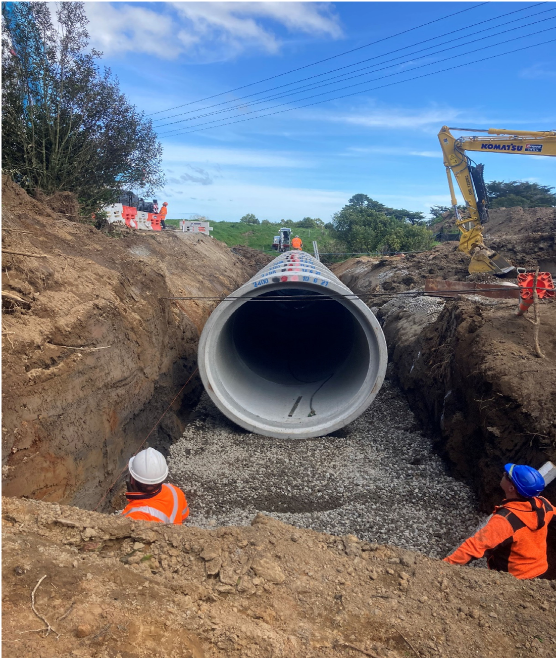
Figure 3: New pipes in the trench across Manaia Rd. Note overhead power lines and underground telecom cables.
