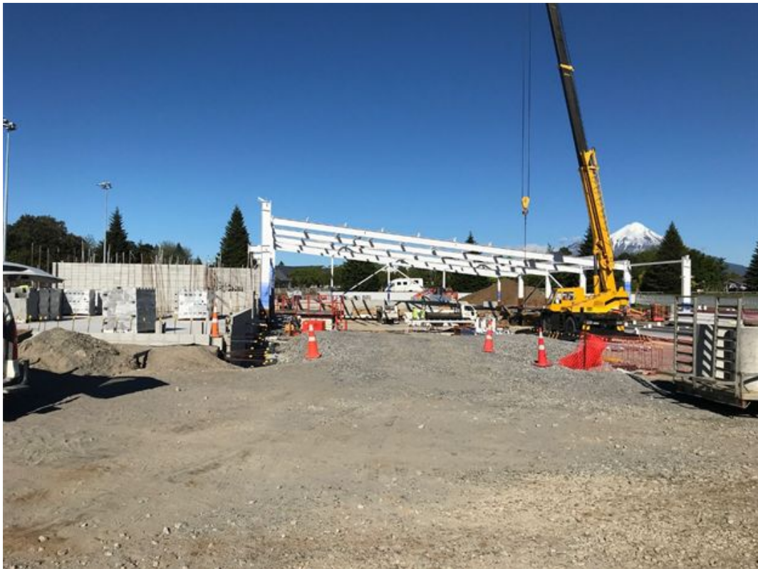
Figure 11: New aquatic centre dryside blockwork completed to height and portal steel under erection
