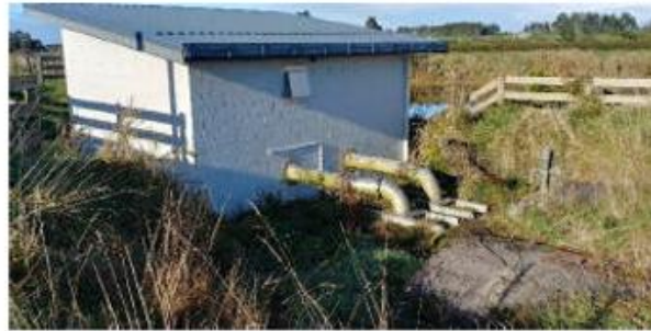
Grit tanks & raw water pump station
