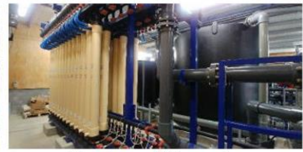
Membrane filter racks
