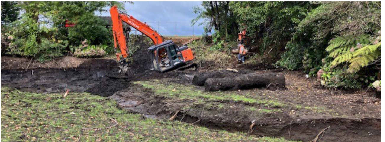
Victoria Park pond was drained and cleaned to look after its health and ensure it continues doing the important job of filtering silt and sediment out of incoming water before the flow joins the Pātea River.
