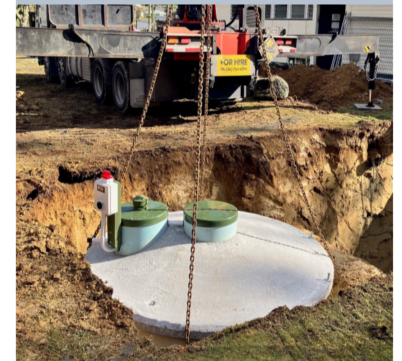
New septic tank at Whangamomona Camp
