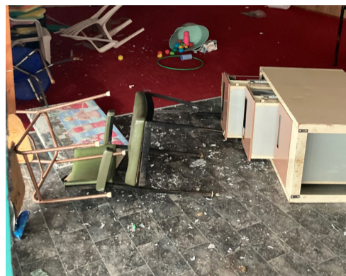
Some of the broken glass and mess left after a recent break-in at the old pool complex.
