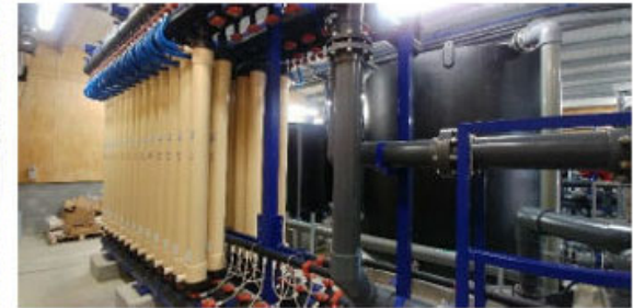
Membrane filter racks
