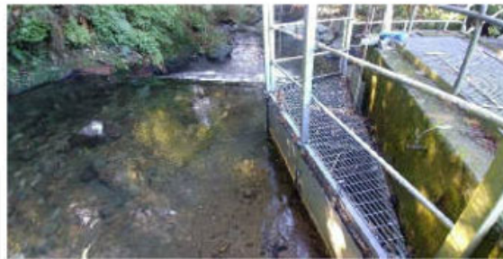
Patea River intake structure
