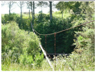
Reticulation supply pipe suspended over the stream
