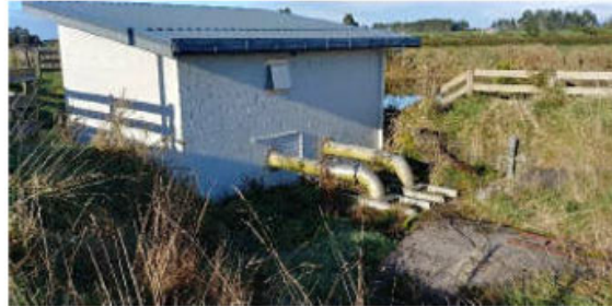
Grit tanks & raw water pump station
