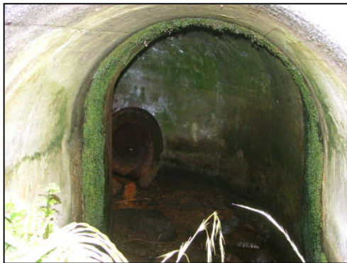
Inner view of pipes and culverts which originally would have fed water wheel
